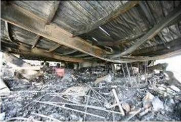
Figure 39 Structural collapse of building
