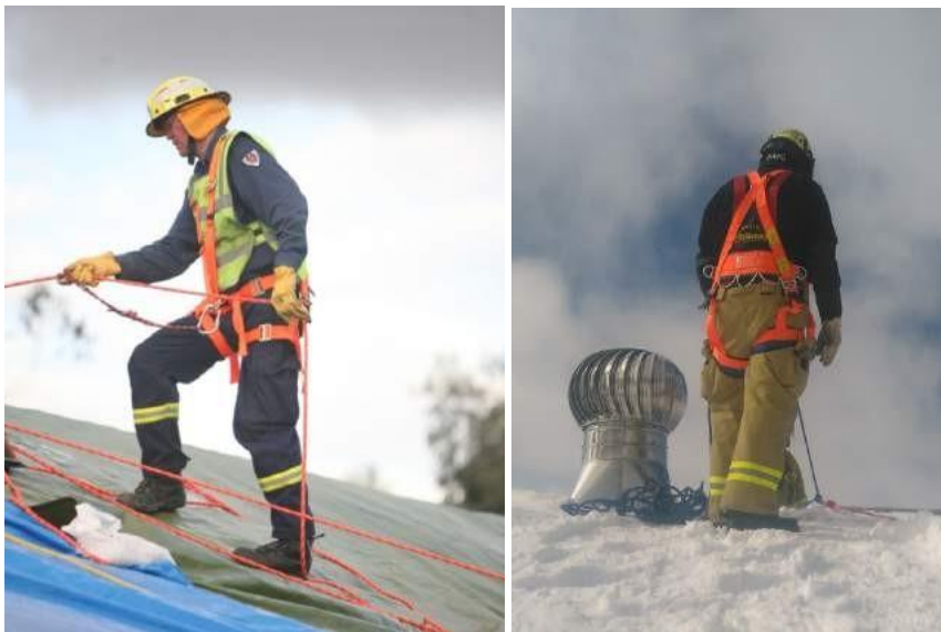
Figure 26 Firefighters working on storm-damaged roofs
